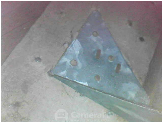
Toe nails - clips with only two nails
