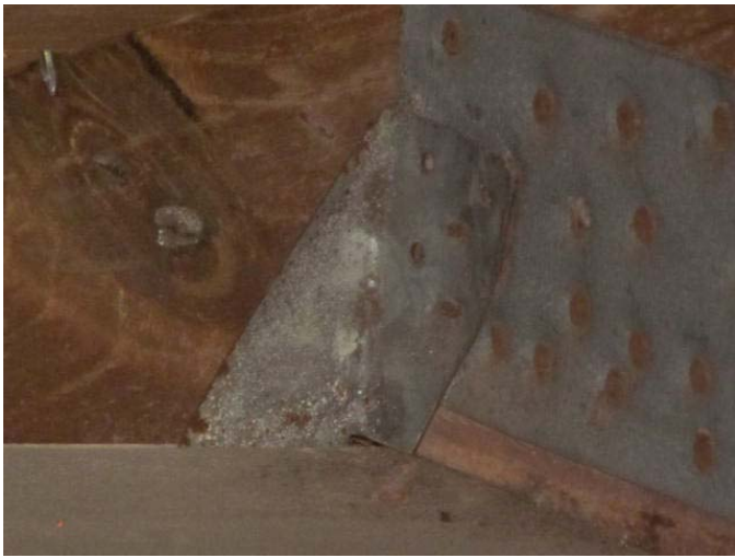
Toe nails - clips with only two nails
