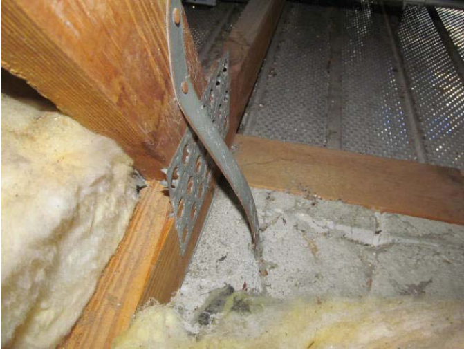
Toe nails - straps further than 1/2"
