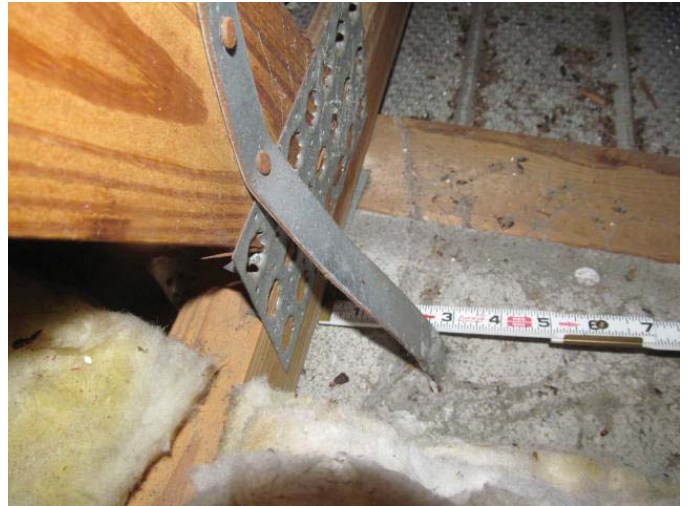
Toe nails - straps further than 1/2"
